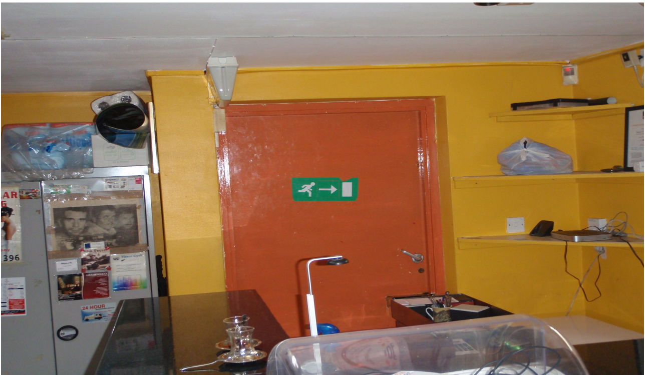
This is the fire exit door at the rear of the room behind the counter. It is intended that this is not used by the public unless in an emergency. The door to remain closed at all times, apart from the occasional use by staff.
